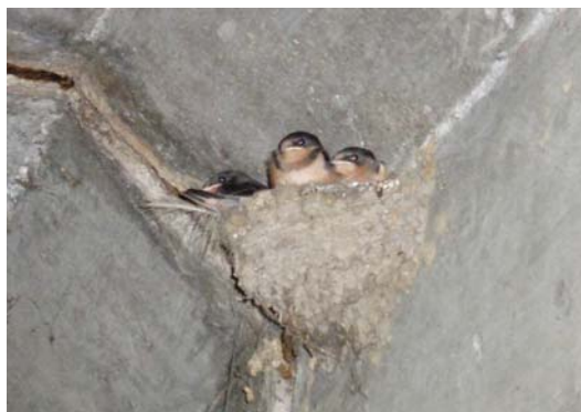
Figure 5-20. Birds Nesting in BRSC Culvert
